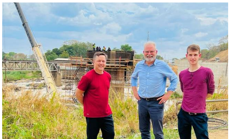
Mr Chrisjan Van Wyk (left) visiting new bridge construction between Kidatu and Mikumi with EcoGraf's Chief Operating Officer Mr Dale Harris and the company's Senior Geologist Mr David Drabble.
