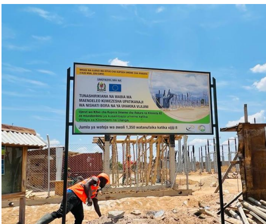
Construction of Ifakara substation a high-voltage transmission line to hydropower stations in Ulanga
